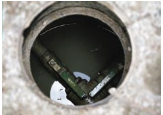
Figure 82—Leaking valve under water.
