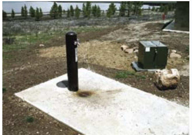
Figure 46—Faucet with concrete pad and drain.
