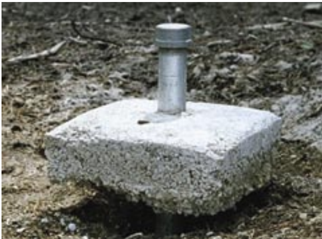
Figure 49—Erosion around vent.
