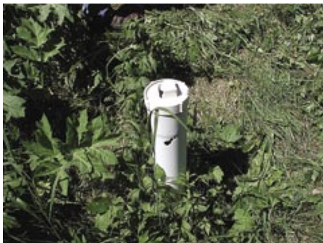
Figure 26—This vent must be repaired.
