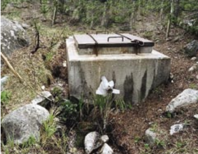
Figure 48—Spring box with erosion damage.
