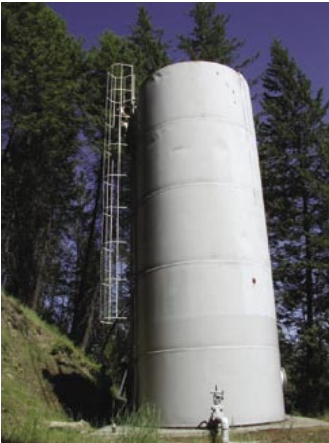
Figure 30—Welded steel water tank.
