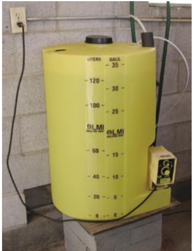
Figure 62—Solution tank and chemical pump.
