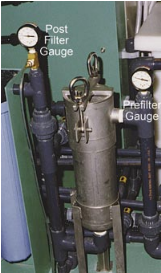
Figure 79—Pressure gauges installed before and after a bag filter.
