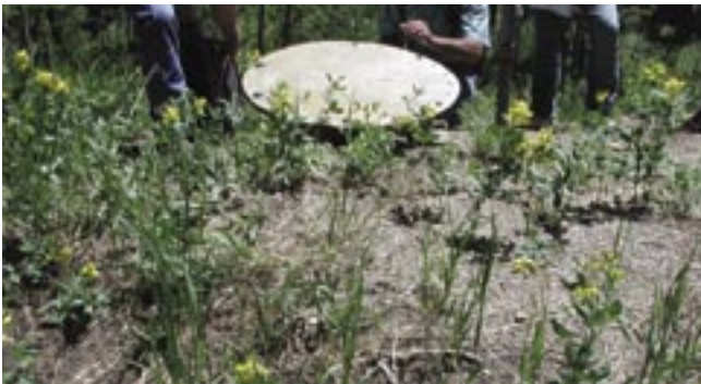
Figure 35—Tank lids must be locked. Replace two opposing bolts with padlocks for security.
