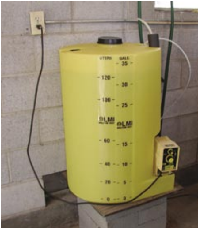
Figure 8—Chlorine solution tank and metering pump.
