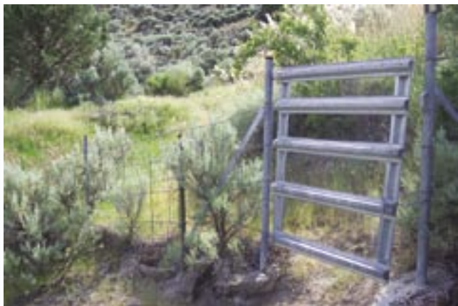
Figure 21—Spring collection area should be fenced and locked.
