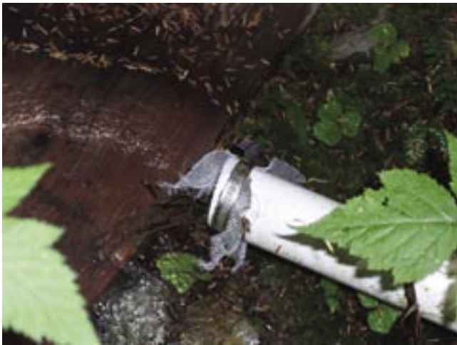
Figure 24—This overflow splash zone is armored. The screen must be repaired.
