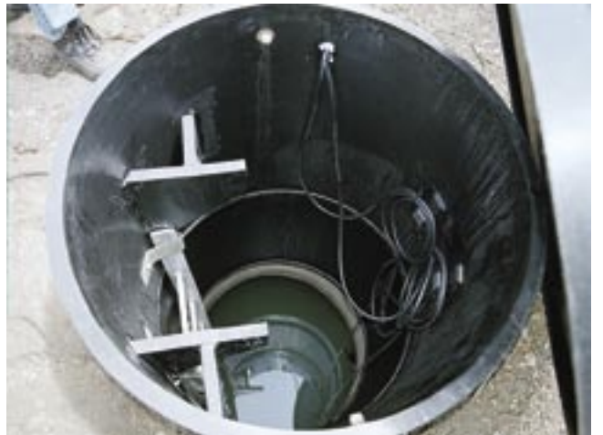
Figure 37—This buried tank access needs a confined space warning and a lock for security.
