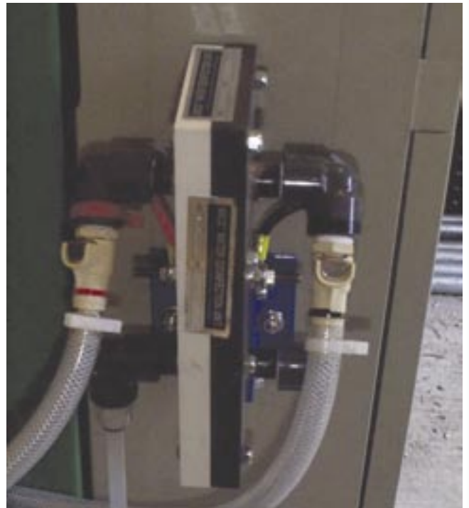
Figure 65—Onsite chlorine generator.
