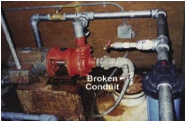
Figure 14—Compromised well seal.
