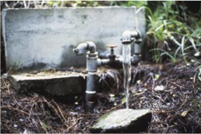
Figure 56—Open winter bypass valve.
