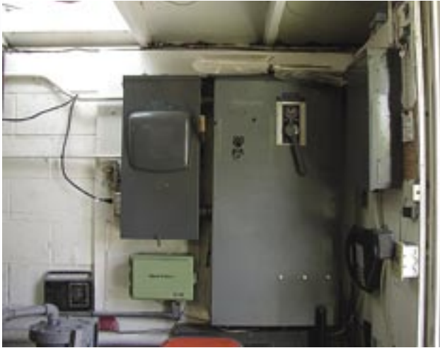
Figure 6—Electrical control panel.
