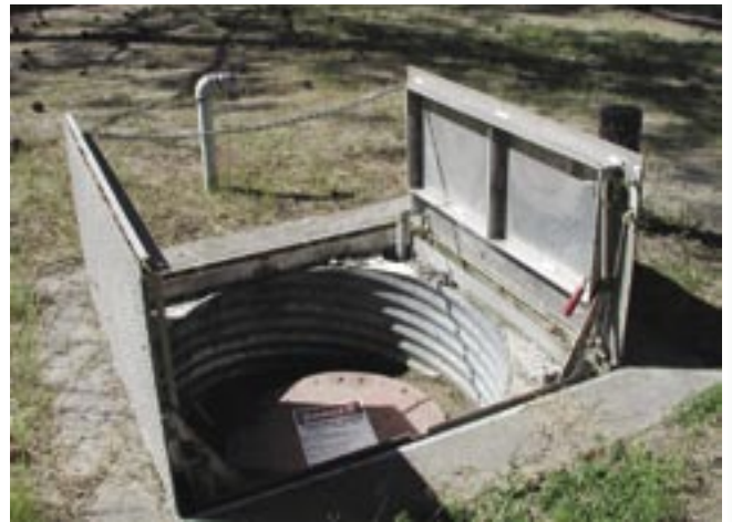
Figure 51—Tanks are confined spaces.
