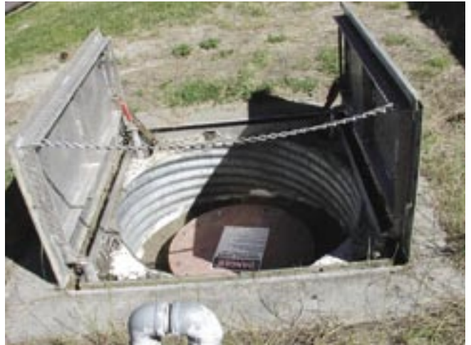
Figure 36—Access to a buried water tank. The outer hatch doors are hinged with a lock. A confined space warning is clearly posted.
