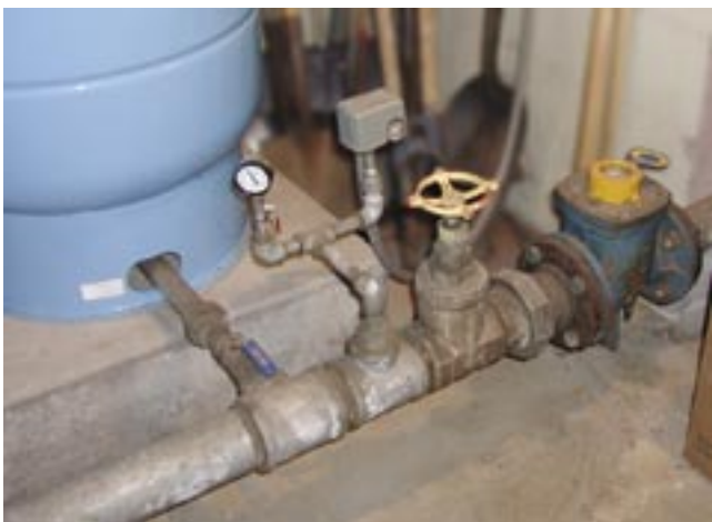
Figure 71—Flowmeter after pressure tank.
