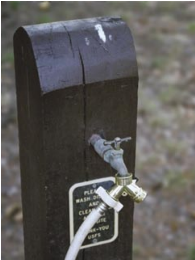
Figure 83—Missing atmospheric vacuum breaker.
