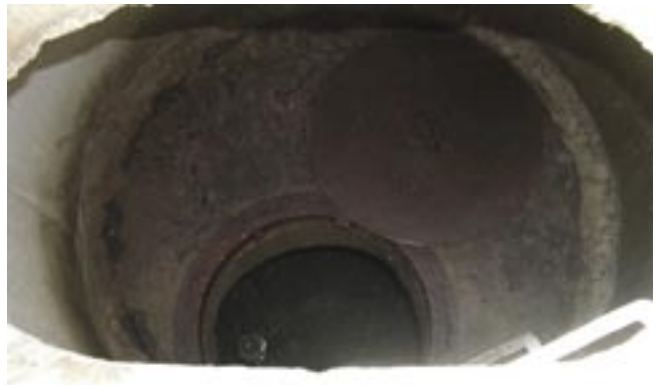
Figure 85—This spring had insects, rust, and debris in the water.
