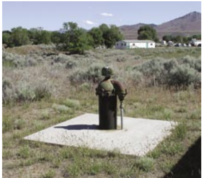
Figure 16—Well pitless adapter with intact slab.
